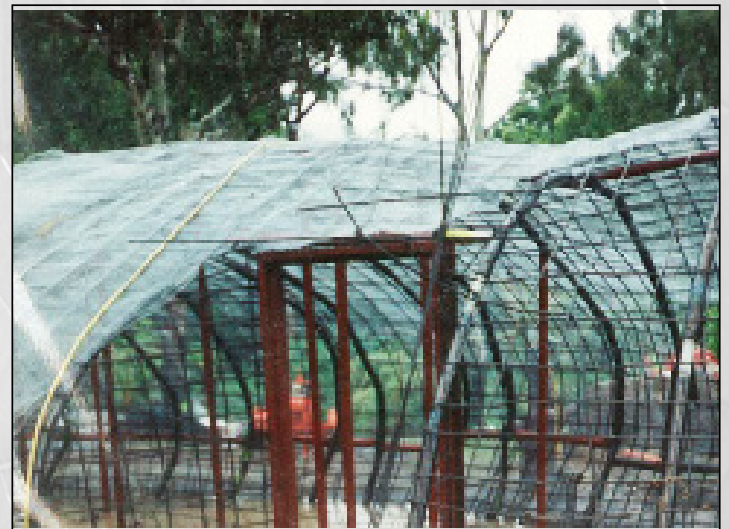
Adding the door frames & application of wire netting over 10mm mild steel bar armature. (It is built in concrete)
