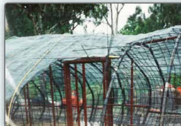
Stage 3 - Adding the door frames & application of wire netting over 10mm mild steel bar armature, which provides the framework for the sturdy concrete finish.
